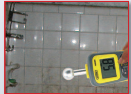
Locate moisture/water damage deep behind tiles
