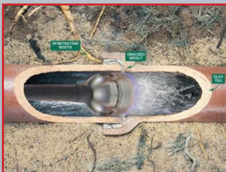
Tree roots cracking and invading a clay sewer pipe
