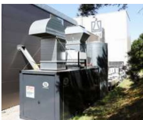
Combined heat and power unit
